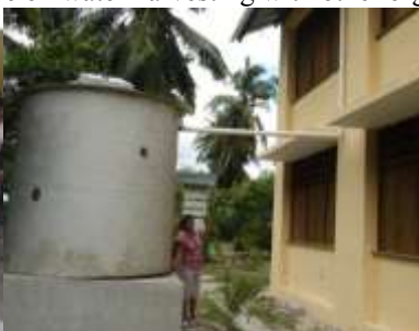
Installed Rainwater Tank
